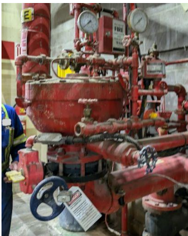
Sprinkler systems that are shut off for maintenance or repairs are a common fire protection impairment
