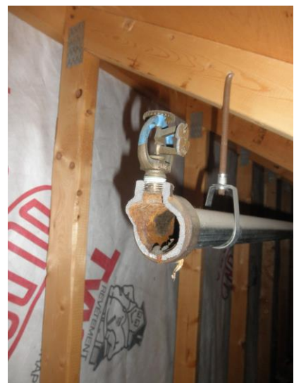
This sprinkler pipe broke due to freezing conditions, creating an impairment until it could be repaired.
